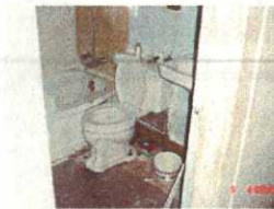
Leaking Faucet/Faulty Plumbing which can lead to mold/mildew
