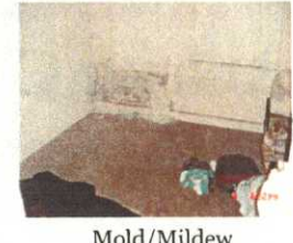
Mold/Mildew Open/Vacant Excessive Trash/Rubbish
